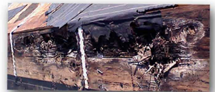
(picture of dryrot due to no attic venting)
